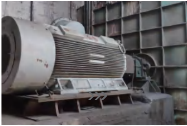
After Retrofit of the 2,500 kW Main Shaft Fan
